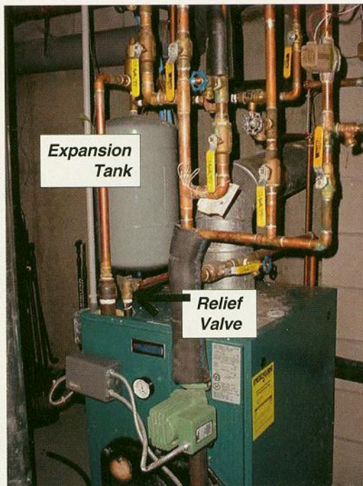
Hot water heating system
