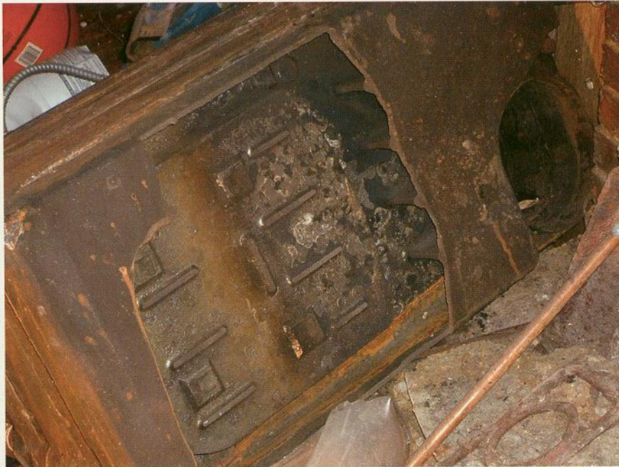
(Above) boiler section damaged due to BLEVE
