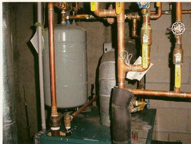
Close up of expansion tank and pressure safety relief valve
